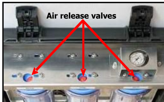
Figure 7: Air release valves on filter housing
